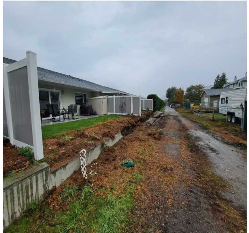
Cedar hedges removed shows how close the cedars were to the homes.
