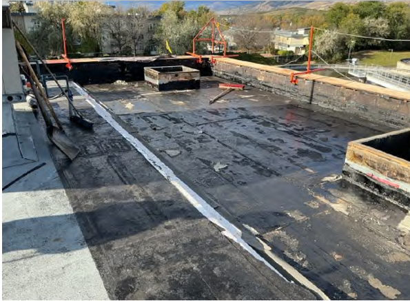
VWRC final section torn off.
