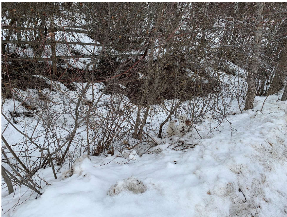
Photograph 10. View of the area around the culvert inlet under snow cover (February 25, 2021).
