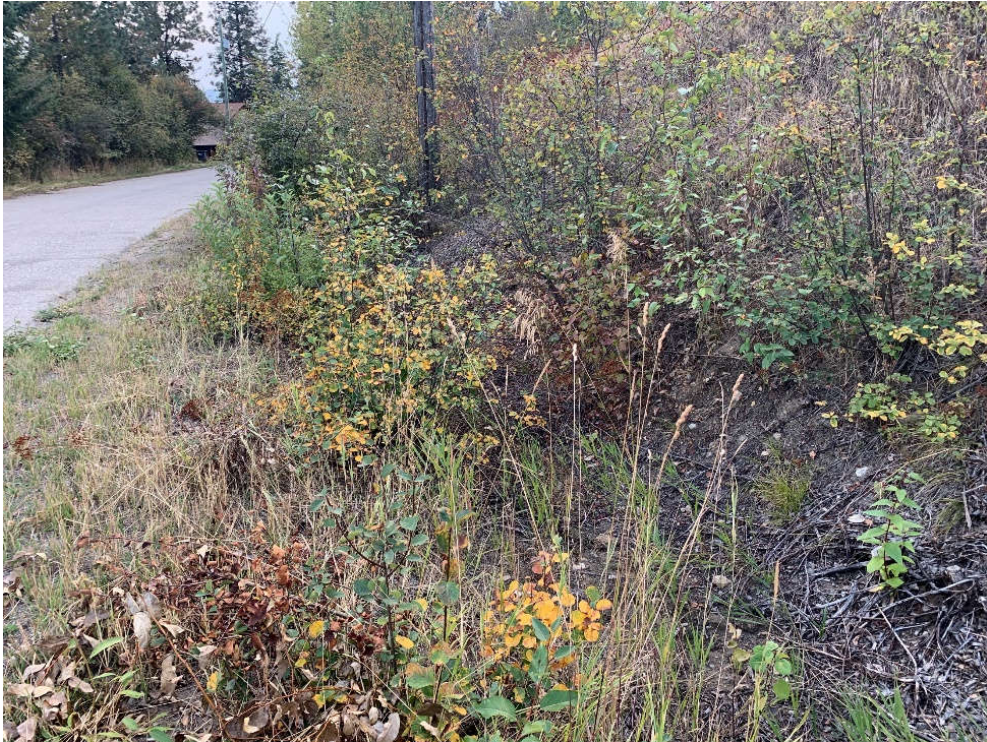
Photograph 15. View south of ditch on the side of Herbert Road. The ditch was dry and overgrown with vegetation during all site visits (September 28, 2022).
