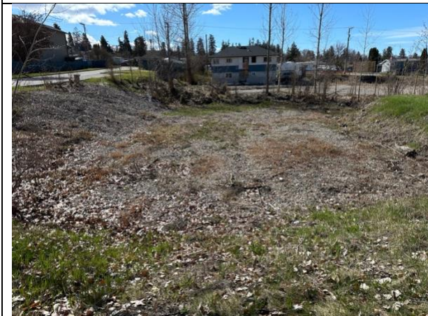
Photo 5: View of the southern excavation west of the ex. Road looking south
