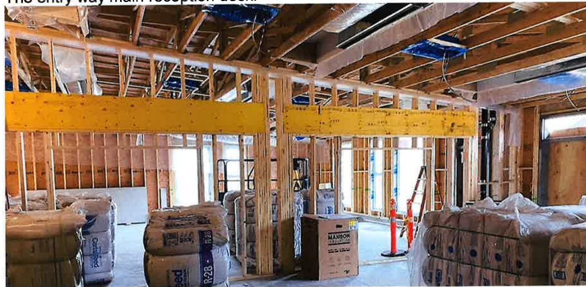
Inside 3-5 room looking into other 3-5 room (HVAC and Lighting are being installed)
