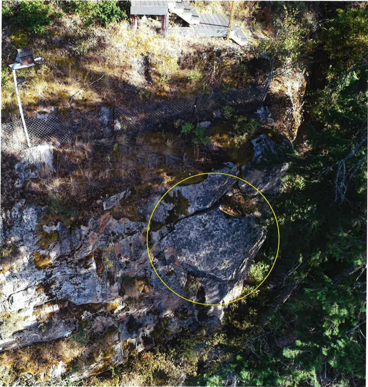
Figure 2. Loose rock block.
